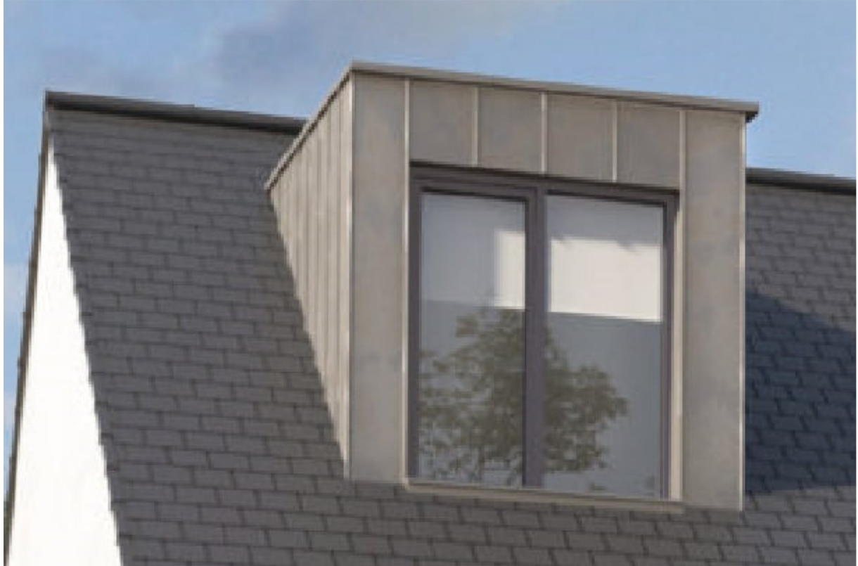
Dark Grey Coloured Pressed Metal Cladding to Contemporary Dormer Elements including uPVC/ aluminium windows
