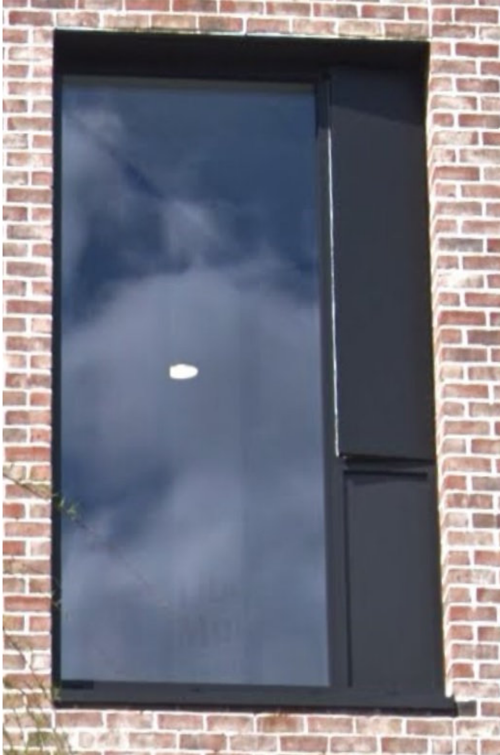
Powder coated grey coloured aluminum/ uPVC windows to facades (set within brick/ render surrounds)
